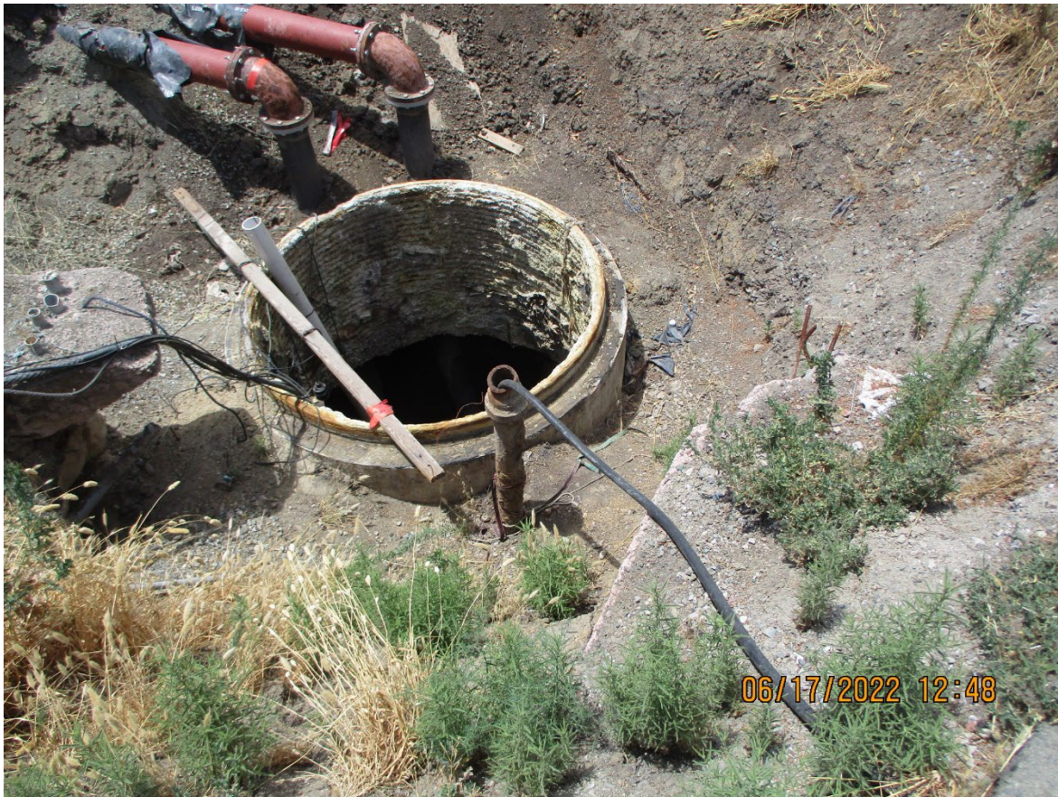
Figure 1 - Pump Station W Currently
