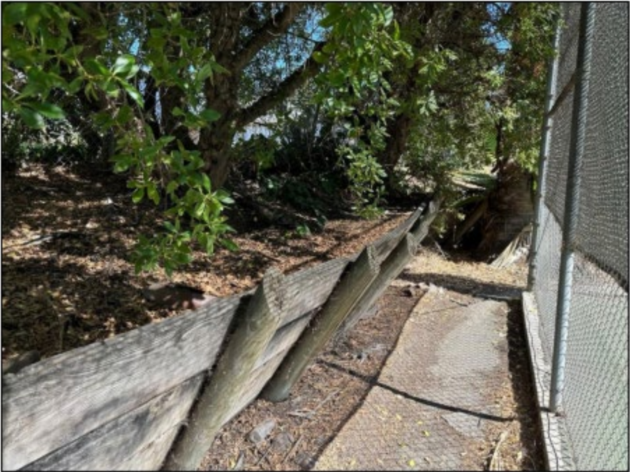
Failed Retaining Wall
