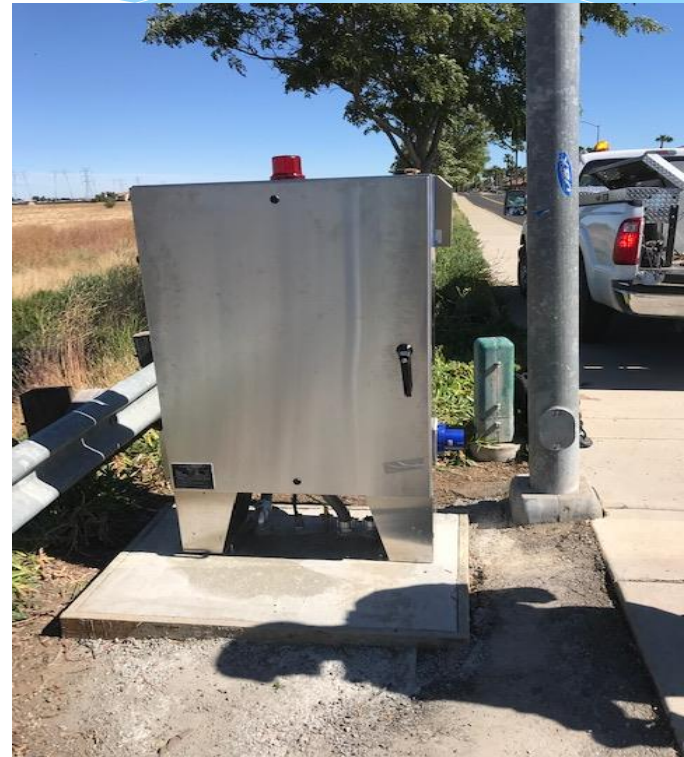
New Control Panel
