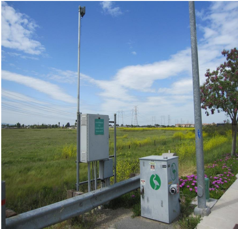
Old Control Panel
