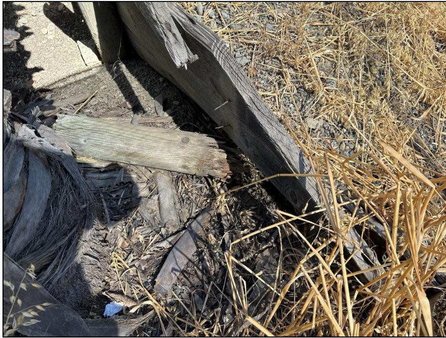
Exhibit 3 – Sheared-Off Wall Post. Rot visible.
