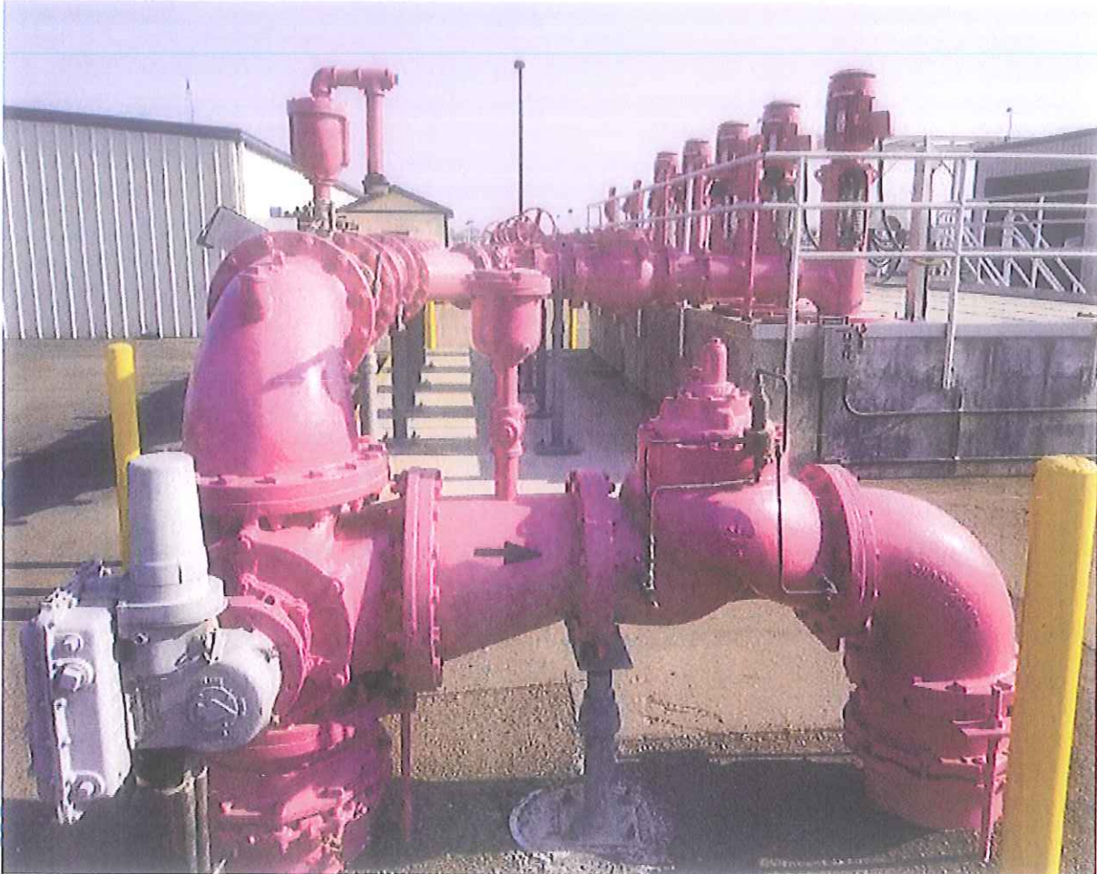
Photo B Discovery Bay Community Service District Sewage Treatment Plant Export Pump Station
