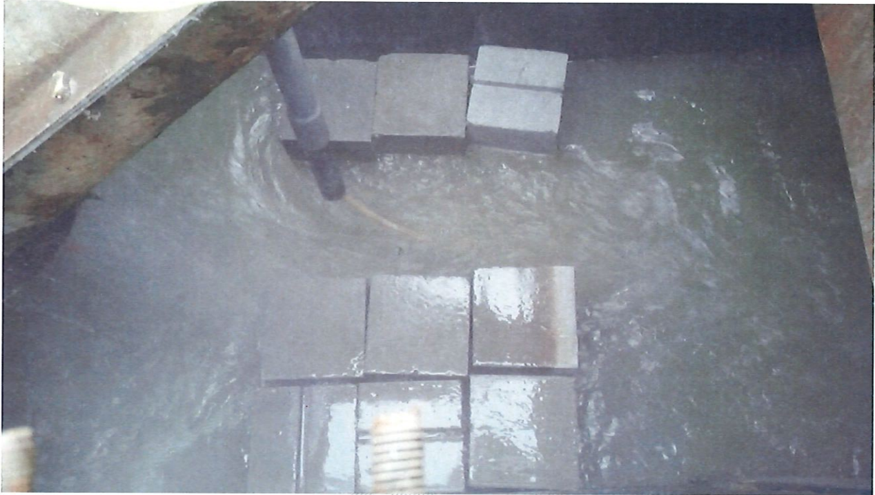
Figure 5-14 Final Configuration of Concrete Blocks and Sampler Intake Tube in Screen Channel on 4-4-2019.
