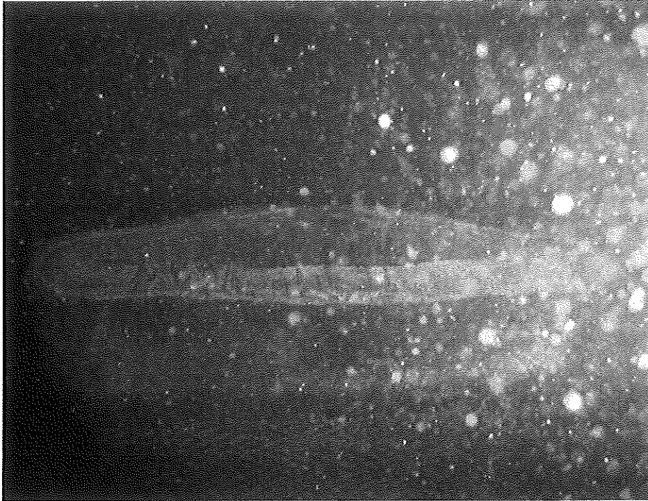
Photo 3 Discovery Bay Outfall Diffuser - Tideflex Valve Showing Crack Damage at its Opening
