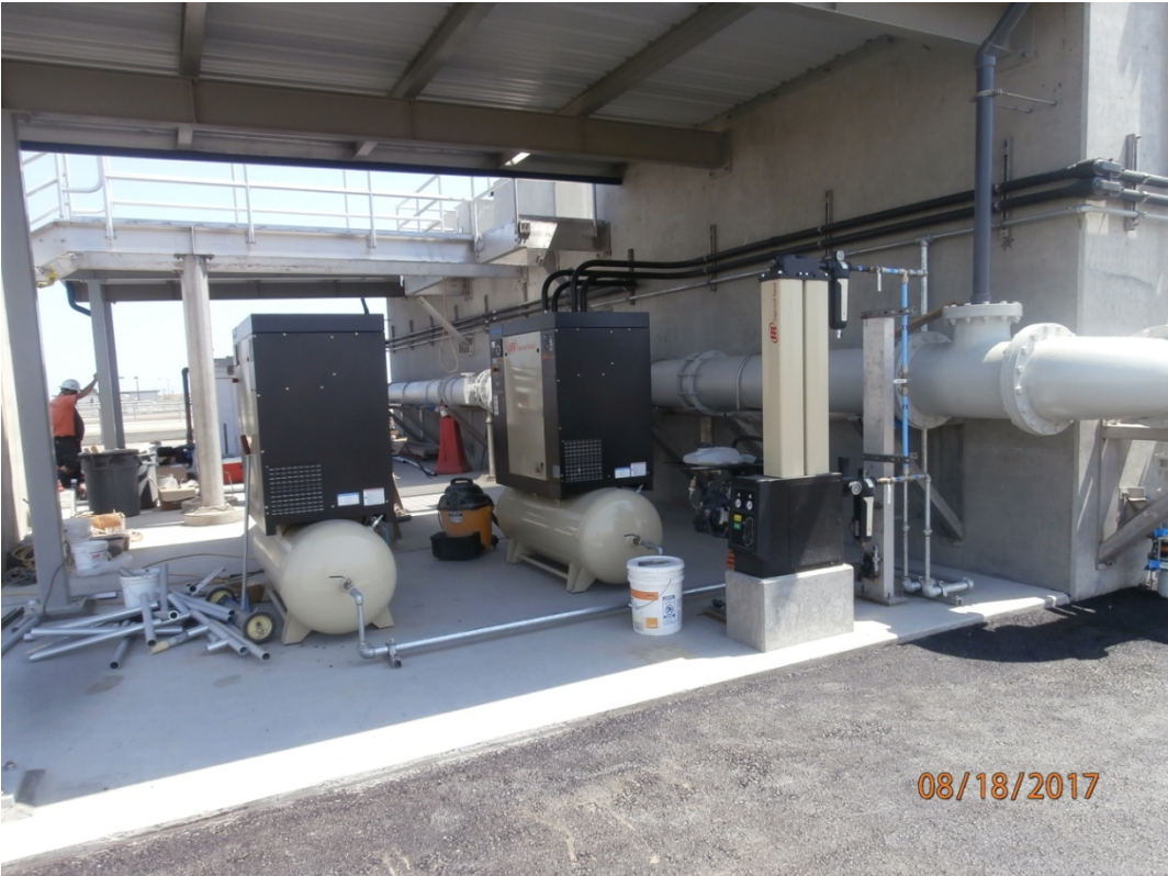
Figure 4 - Air Compressors for Filter System
