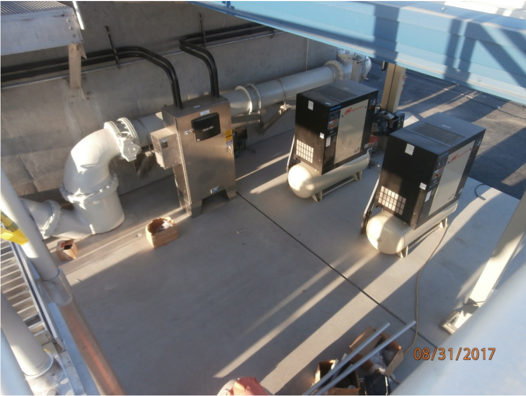
Figure 3 - Filter Control Panel and Air Compressors
