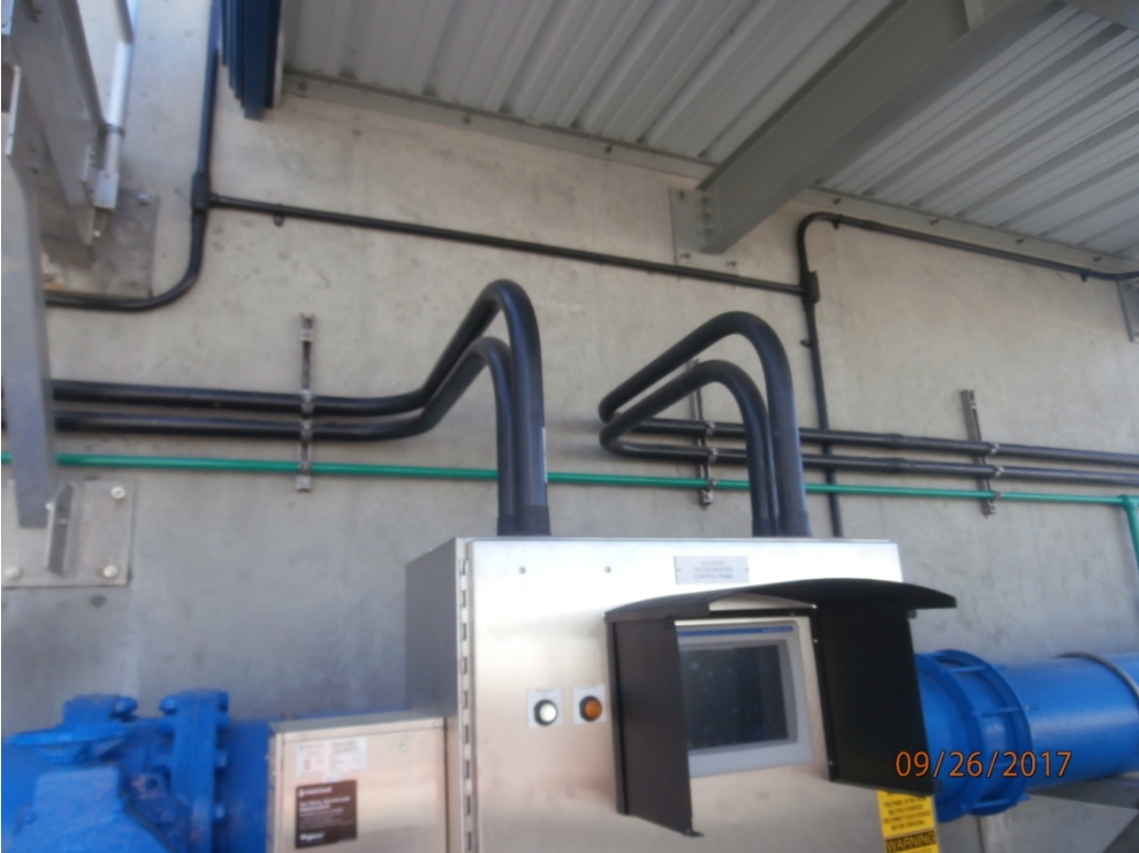
Figure 5 - Filter Control Panel
