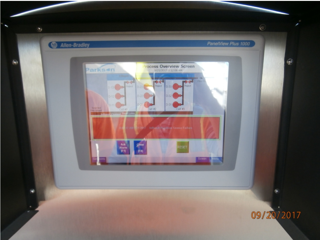
Figure 6 - Filter Control Panel Controls Operation of the EcoWash Feature Which is Selectable From the Main Control Screen.
