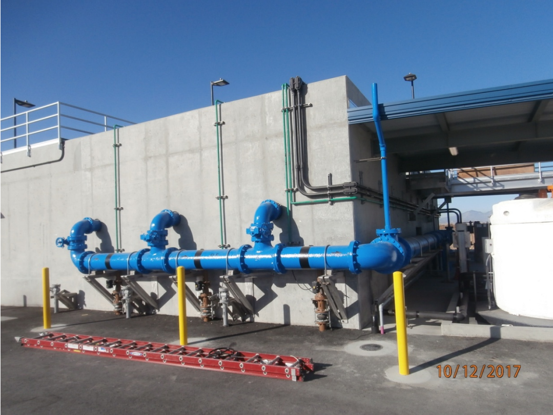
Figure 1 - New Filter System at the Town of Discovery Bay
